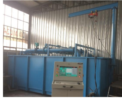
Şekil 4 Pompa test sistemi Figure 4 Pump testing system
