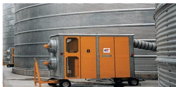
Figure 5. GRANIFRIGOR™ grain cooling in steel silos (Brunner, 1989)
